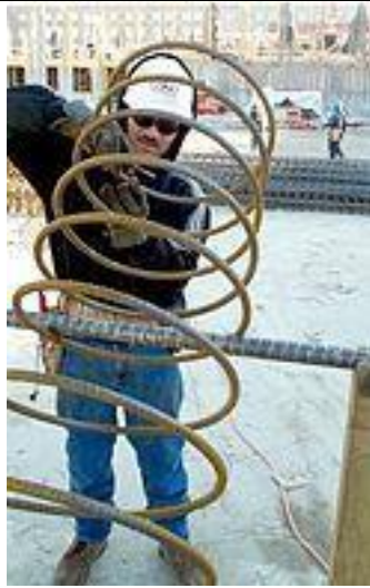
Fig. 5. A steel fixer wears protective gloves while handling a coil of rebar, which will be embedded in a reinforced concrete column to strengthen it.
