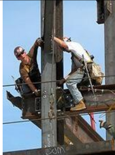
Fig. 6. Ironworkers are erecting the steel frame of a new building at the Massachusetts General Hospital in the United States.
