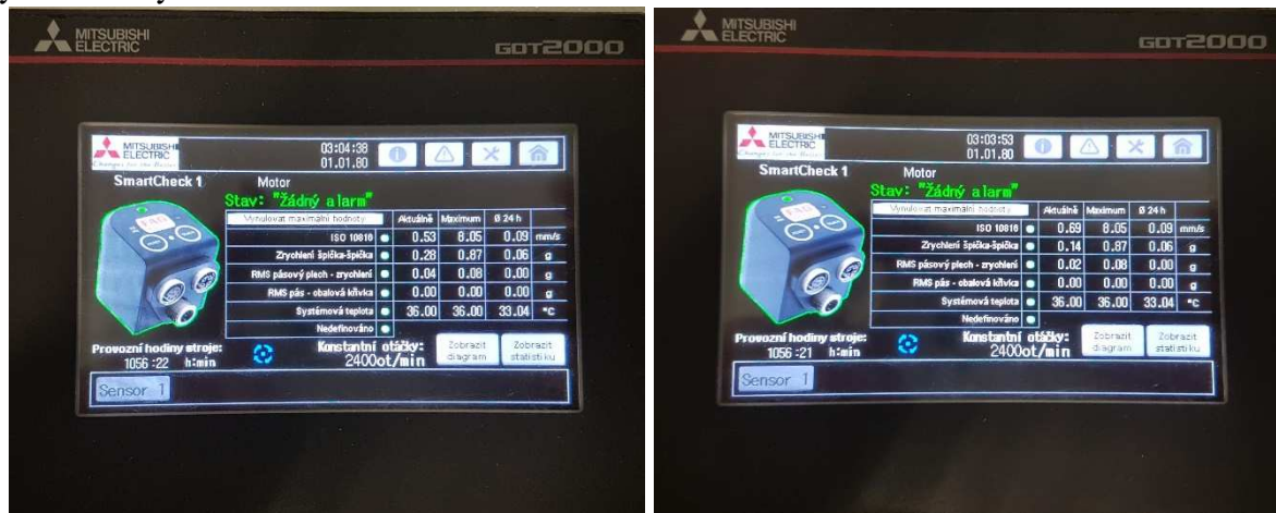
Fig. 8. HMI of Motor 1 and Motor 2 measurements
