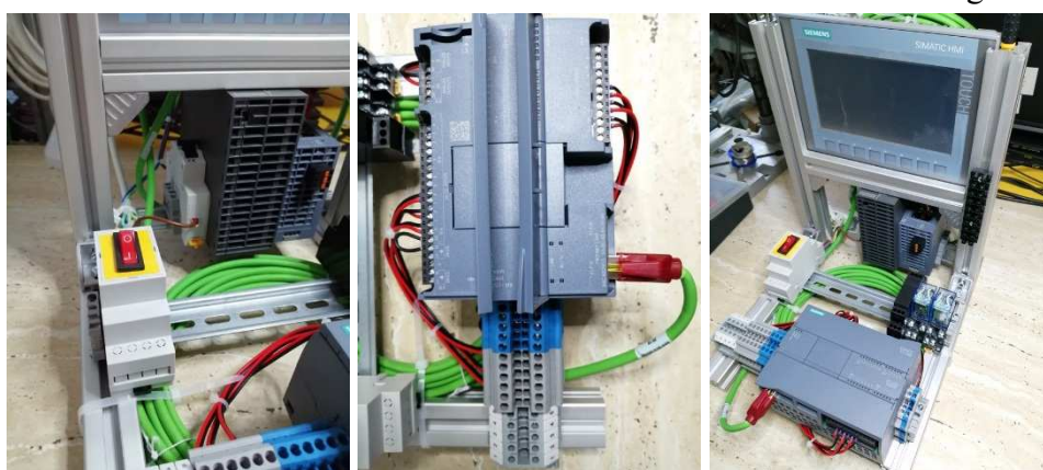
Fig. 7. Total red highlighted power switch (left); additional screw terminal (middle); Profinet switch (right)
