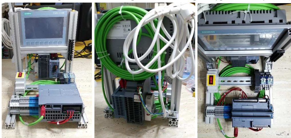
Fig. 6. Training PLC stand overall configuration (left); back side of stand with power supply and circuit breaker (middle); upper view to stand (right)
